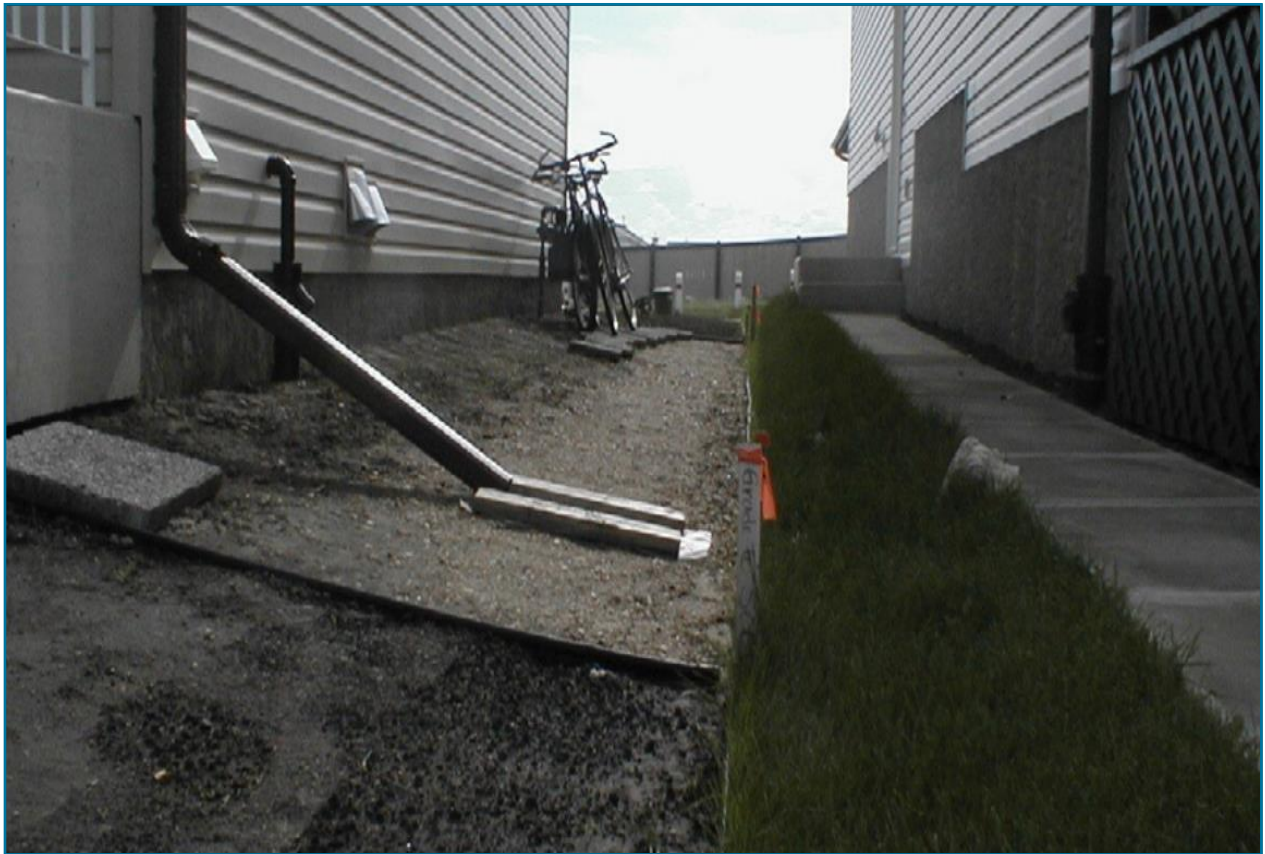
This rough grade base has been raised to match the final grade before placing decorative rocks. Ponding will potentially be minimized.
