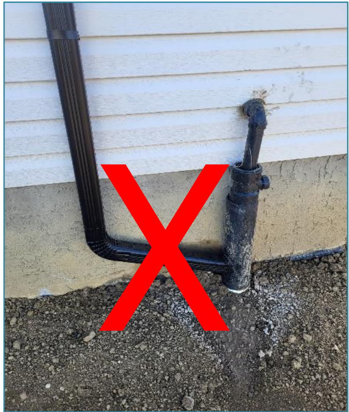
Downspout incorrectly connected to sump pump discharge
