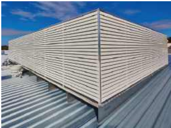
Rooftop mechanical units are screened from view.
