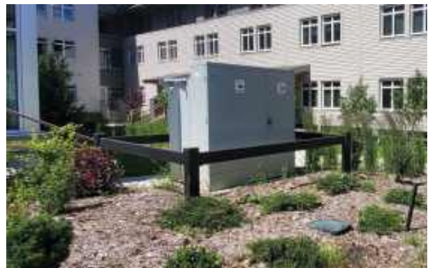
Utility boxes can be installed in the back courtyards of larger developments and integrated with a variety of compatible plantings.
