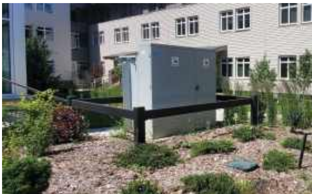
Utility boxes can be installed in the back courtyards of larger developments and integrated with a variety of compatible plantings.
