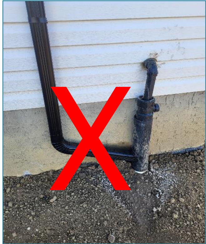
Downspout incorrectly connected to sump pump discharge
