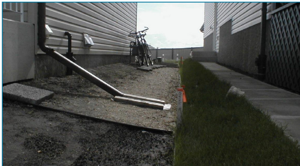
This rough grade base has been raised to match the final grade before placing decorative rocks. Ponding will potentially be minimized.
